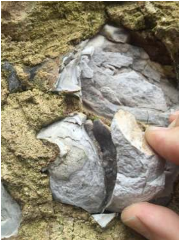
View of Fractured Flint in West Wall
