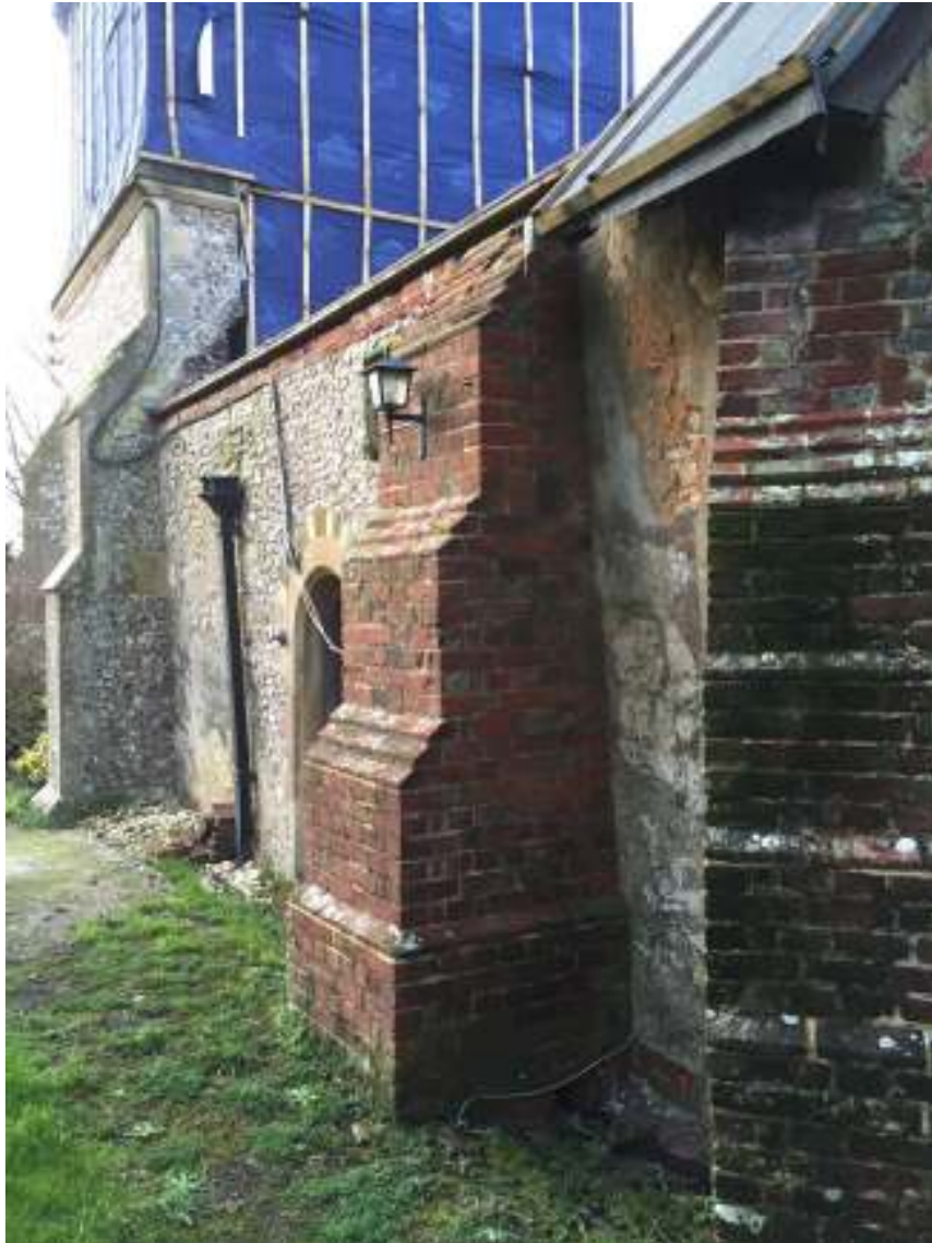
View of The East Section of South Wall Externally – Showing Out of Plumbness
